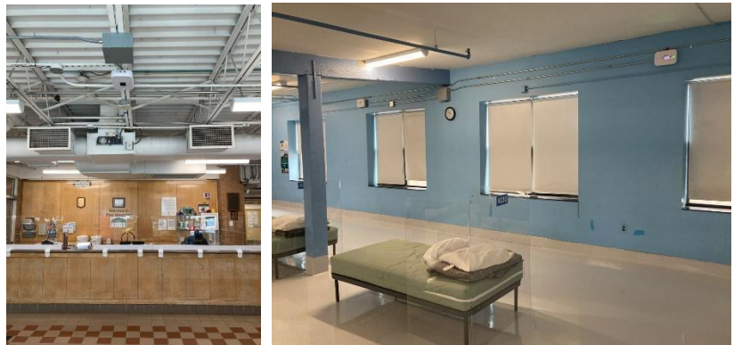
Figure 1 Pine Street Inn WR UVGI fixtures on the ceilings and walls in dormitories, bathrooms, dining and communal spaces. (Source: Equity Air member PJ Piper, Far UV Technologies)
